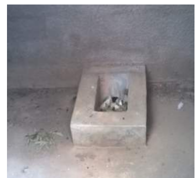
Figure 34: Clogged latrine at Nacacane Health Centre.
