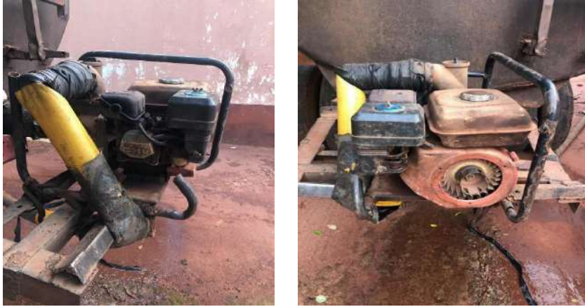
Figure 7a,b:Picture of household pump located at Eze-Opi; UNN
